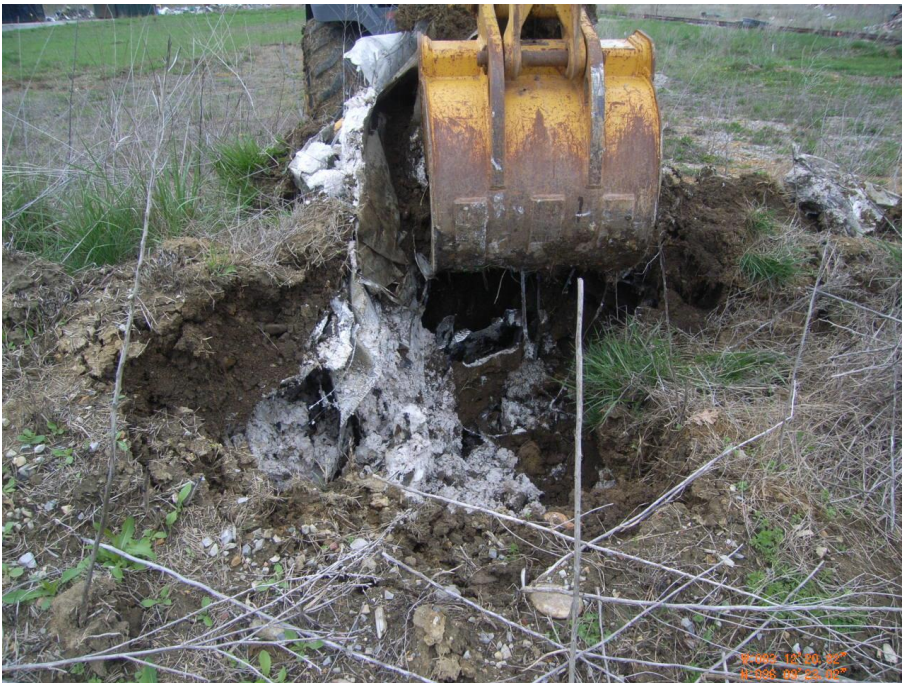
Buried asbestos intermingled with other demolition debris
