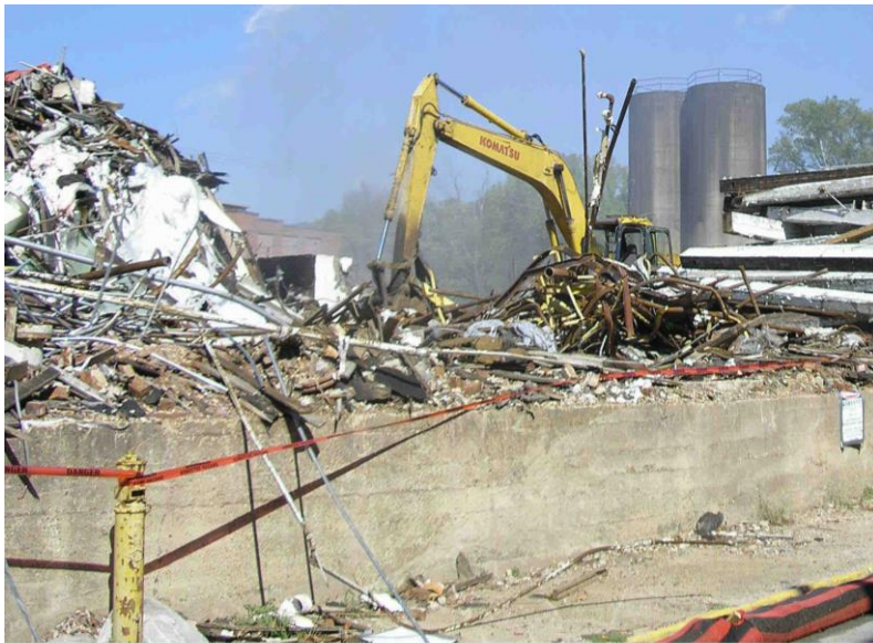
Example of unlawful asbestos demolition
