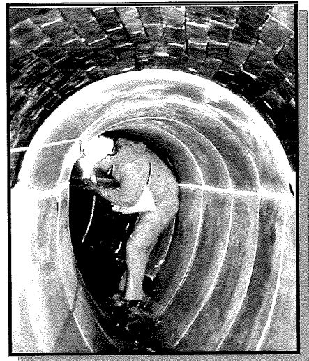
Sewer rehabilitation can include lining aging sewers (photo: NJ Department of Environmental Protection).
