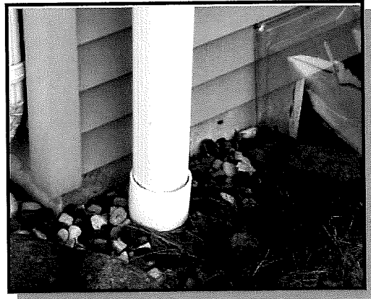
Sources of stormwater in the collection system may include building downspouts connected directly to the system (photo: MMSD).
