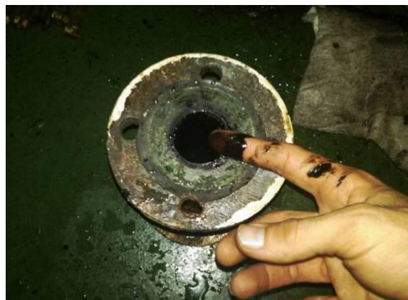
Overboard discharge with oily residue
