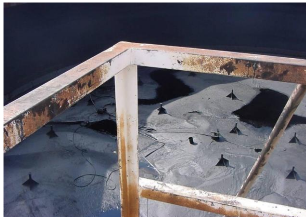
Oil on rooftop
