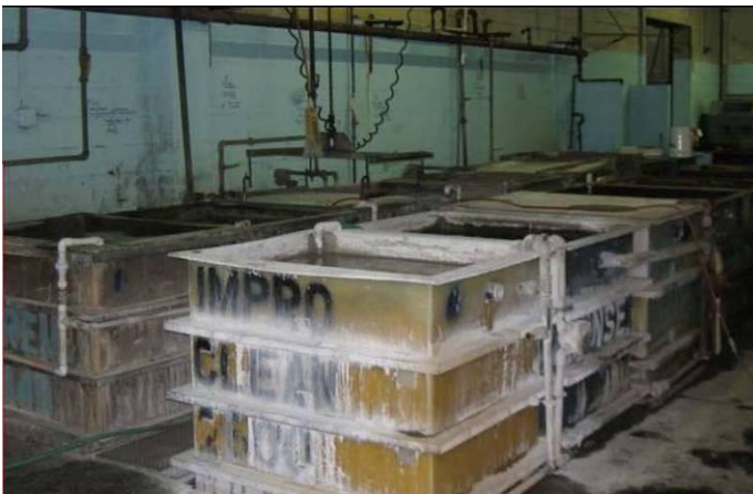
Process wastewater overflowing the holding tanks and draining to sewer
