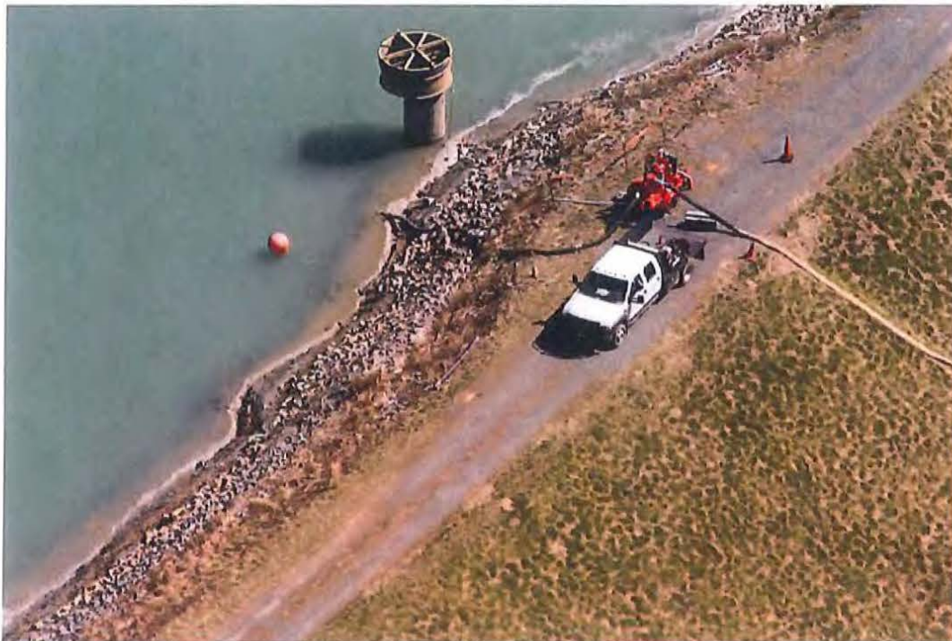
Photograph 10. 3/11/14 aerial photograph of CAPE FEAR 1985 coal ash basin with Godwin pump and truck.
