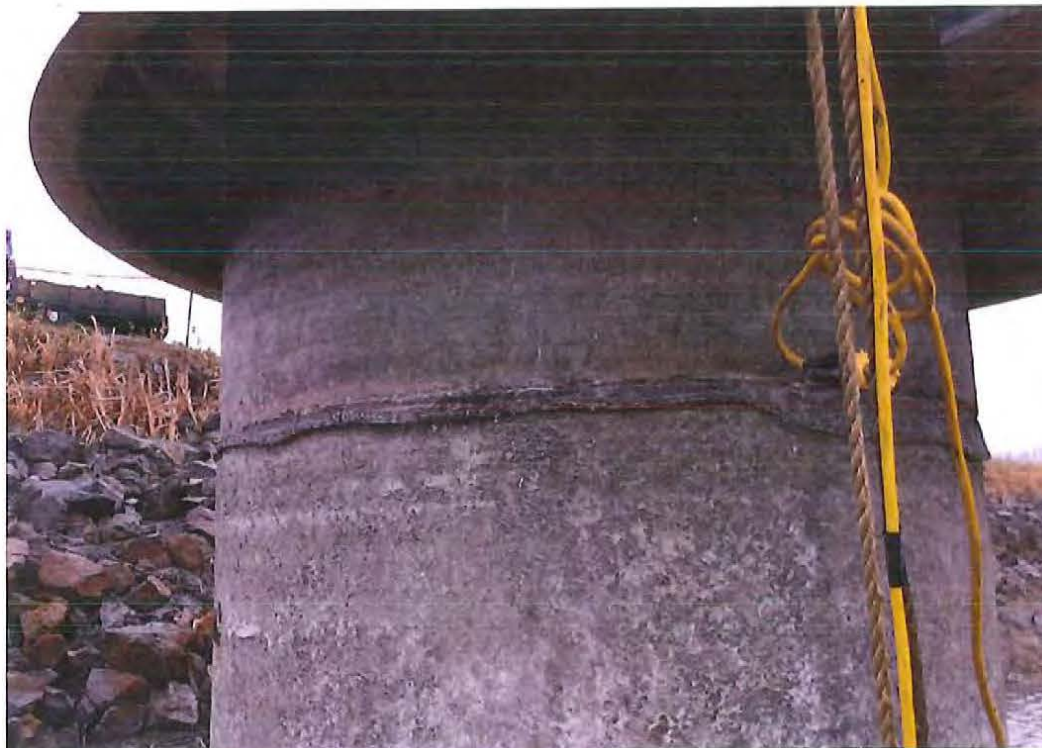
Photograph 13. 3/19/14 photograph of old grout on CAPE FEAR coal ash basin riser.
