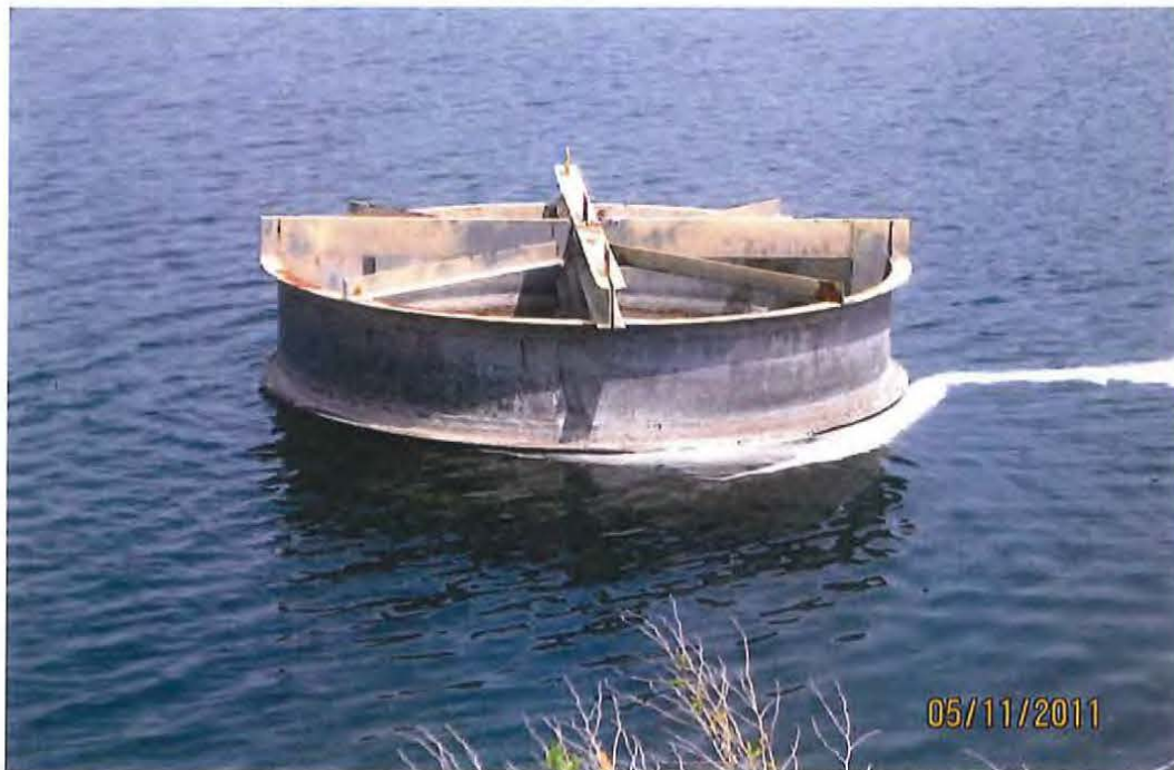
Photograph 7. Riser in CAPE FEAR 1985 coal ash basin from 2012 Five Year Independent Consultant Report.
