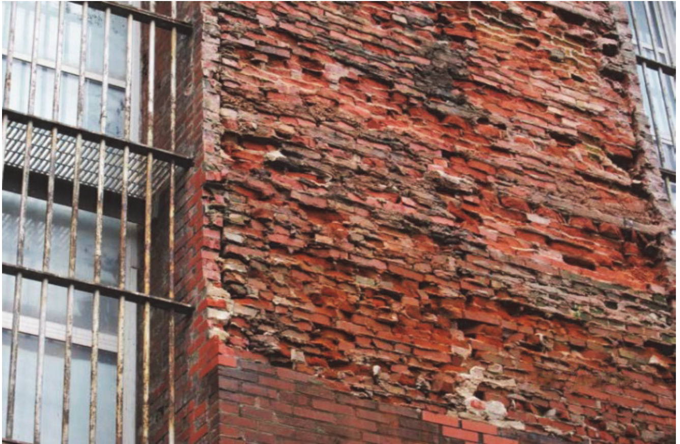
Deteriorating brick wall on Cell House United States Penitentiary, Leavenworth Kansas
