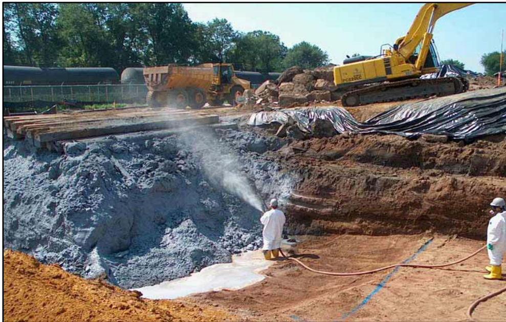
Soil excavation and clean up at a Superfund site, Environmental Protection Agency
