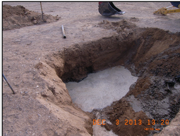
Raw sewage injected underground
