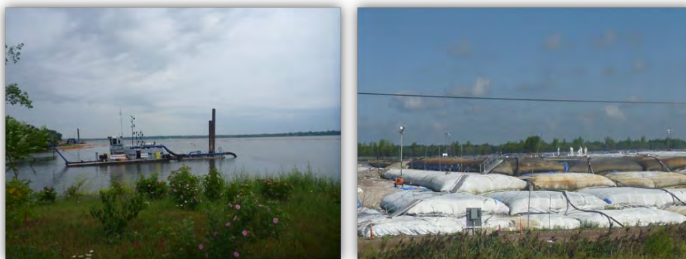
Dredging boat in Onondaga Lake and bags of dredged sediment in wastebed.
