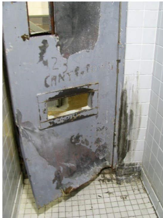
Damaged shower door in a housing unit at a GDC men's prison in 2023.
