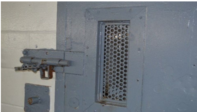
Engaged padlocks on restrictive housing unit cell doors in a close- security GDC prison in 2022. An officer at this prison later told DOJ that padlocks are not used on cell doors at this prison.
